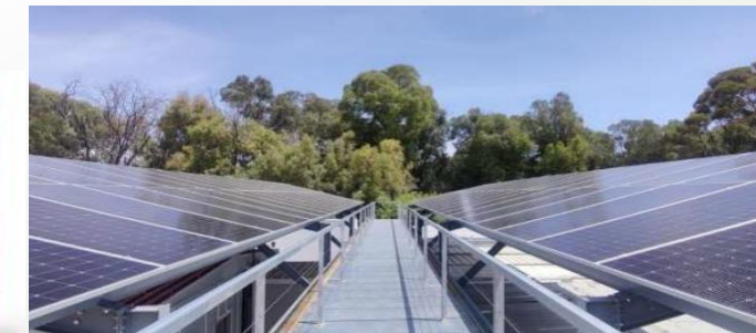
Living Lab - Smart energy microgrid
